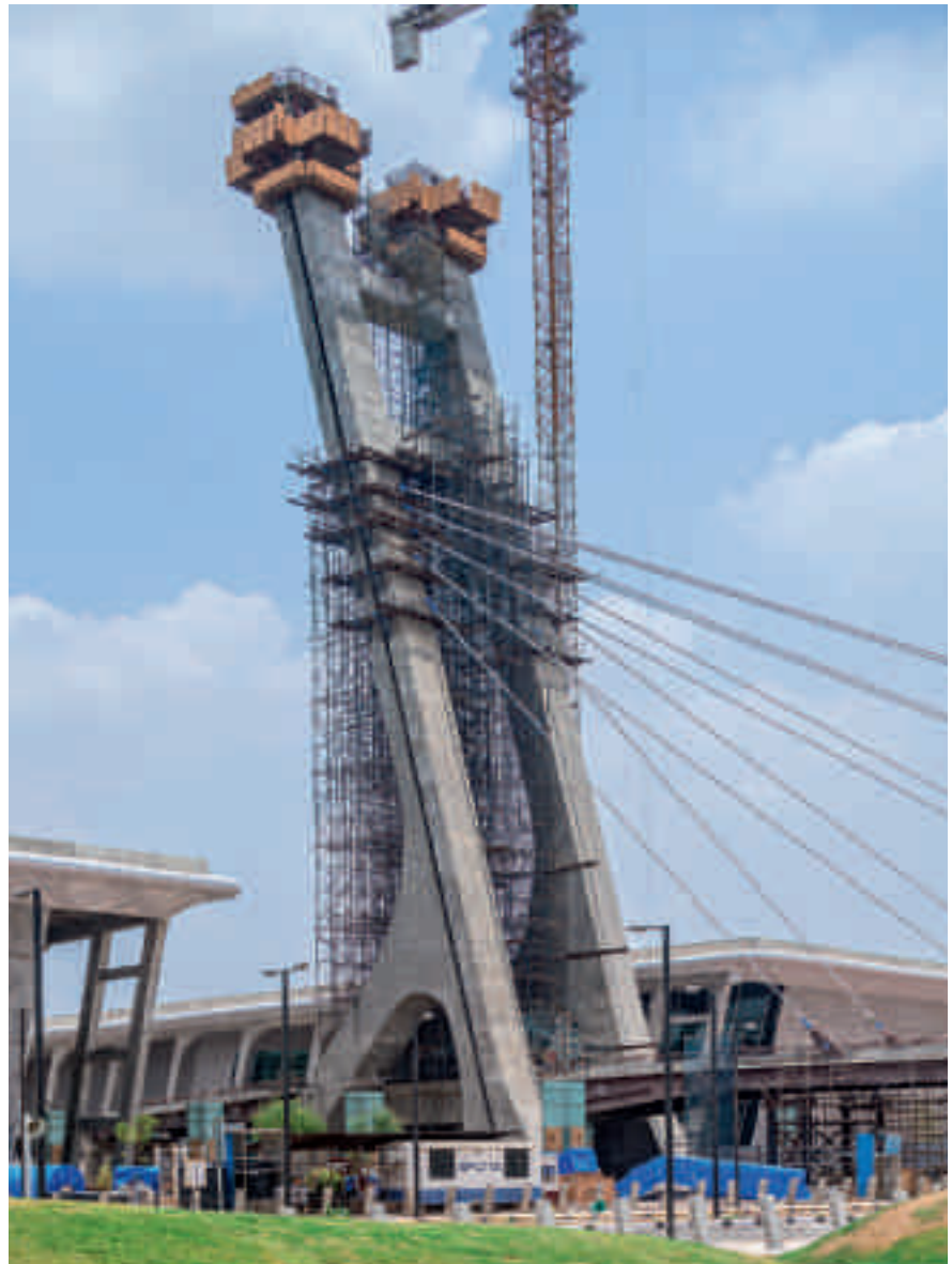
Spacious and safe working areas on all 3 levels.
