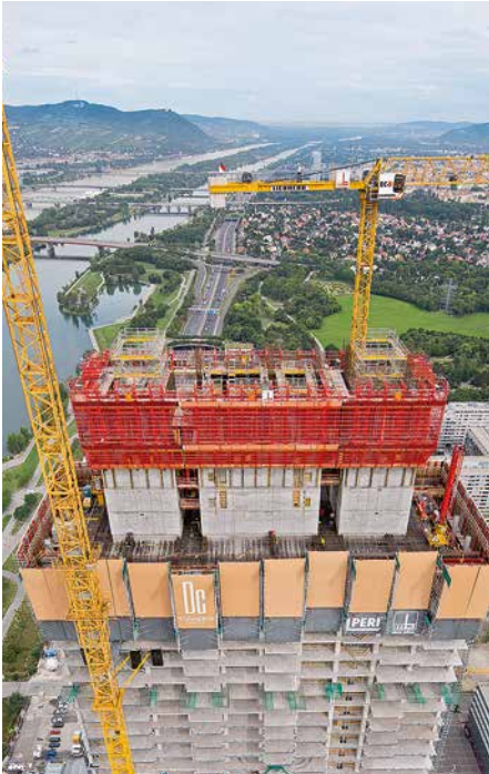
The repeatedly recessed facade construction characterizes the DC Tower in Vienna. The Climbing Protection Panel could be continually adjusted to match the variable floor areas.
